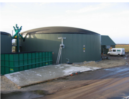
Biogas plant in Twist, Lower Saxony
